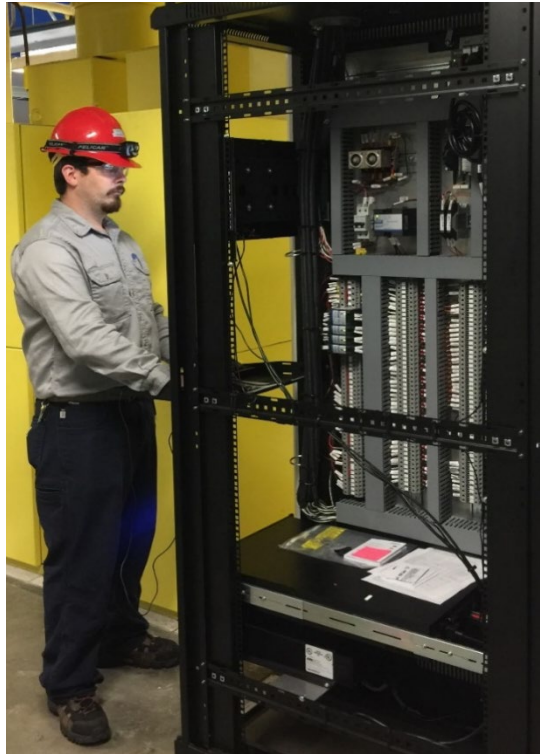
Figure 2 MCM2 installation in rack mount cabinet.
