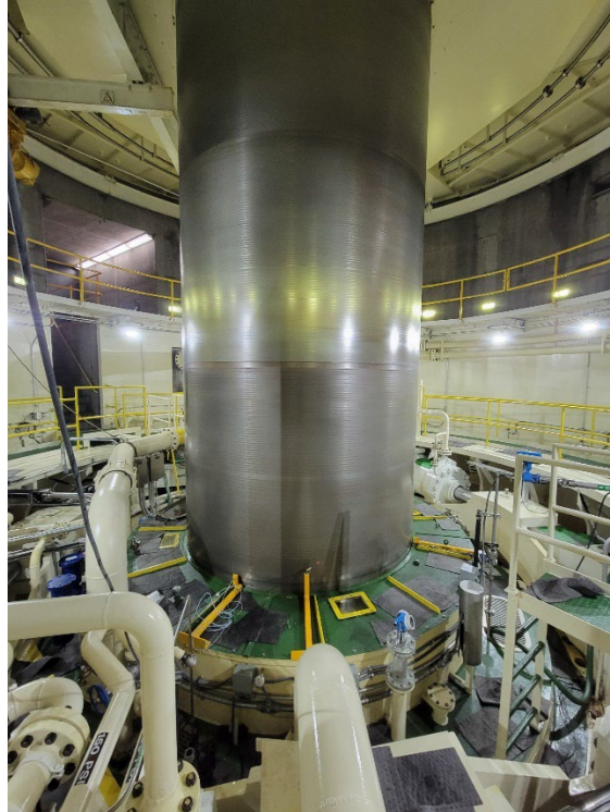
Figure A 2 Typical MCM turbine guide bearing proximity sensors and laser tachometer installation.
