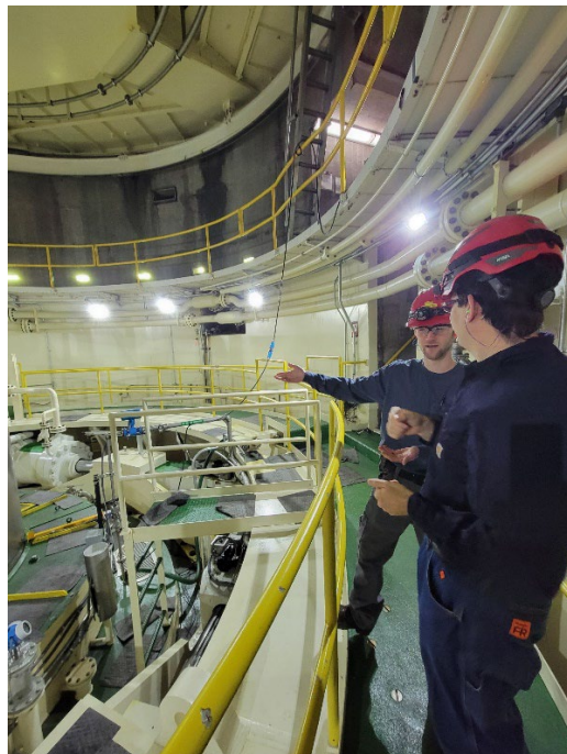
Figure A 3 Discussing MCM monitoring features in turbine pit of current MCM2 installation.
